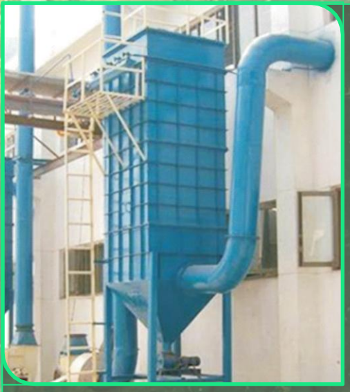
Air Pollution Control Devices
